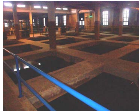
In 2003 rehabilitation of our filter beds will optimize water treatment
